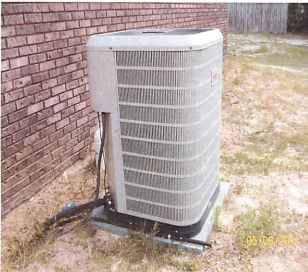
A/C PAD (RIGHT) SIDE VIEW TAKEN 05-09-11
