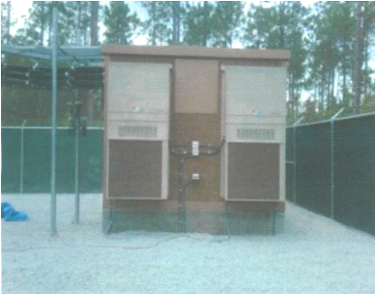
Back of Building with A/C units
