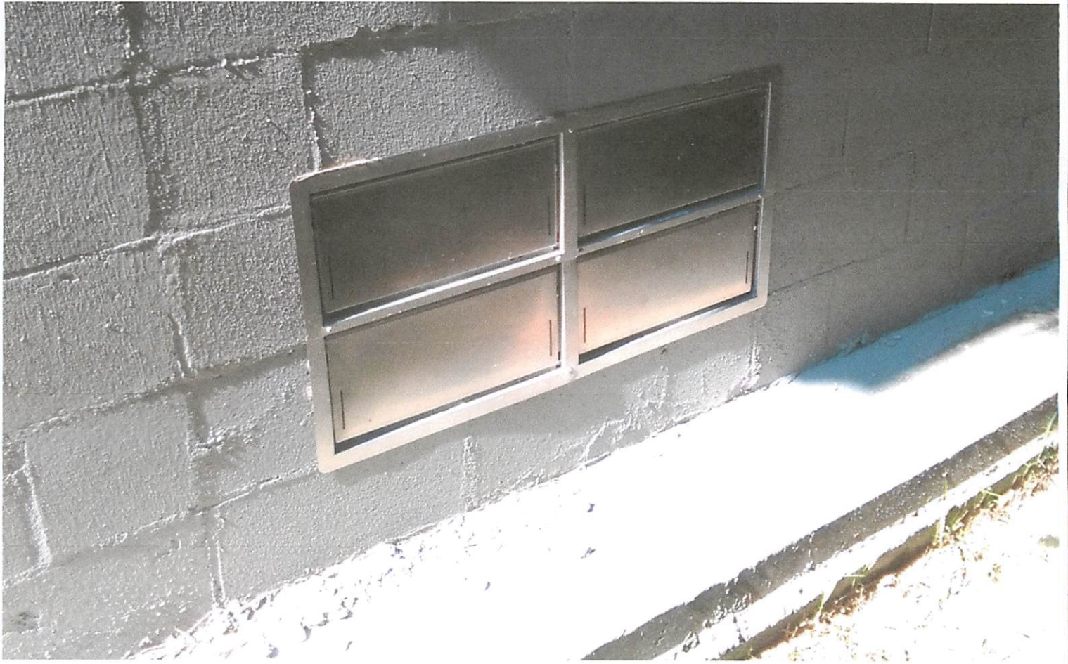
FLOOD VENTS LEFT SIDE VIEW 7/21/2015
