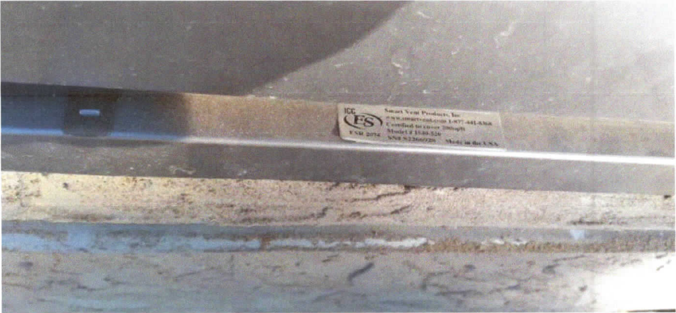
SMAT VENT FLOOD VENT IDENTIFICATION 10-19-2022
