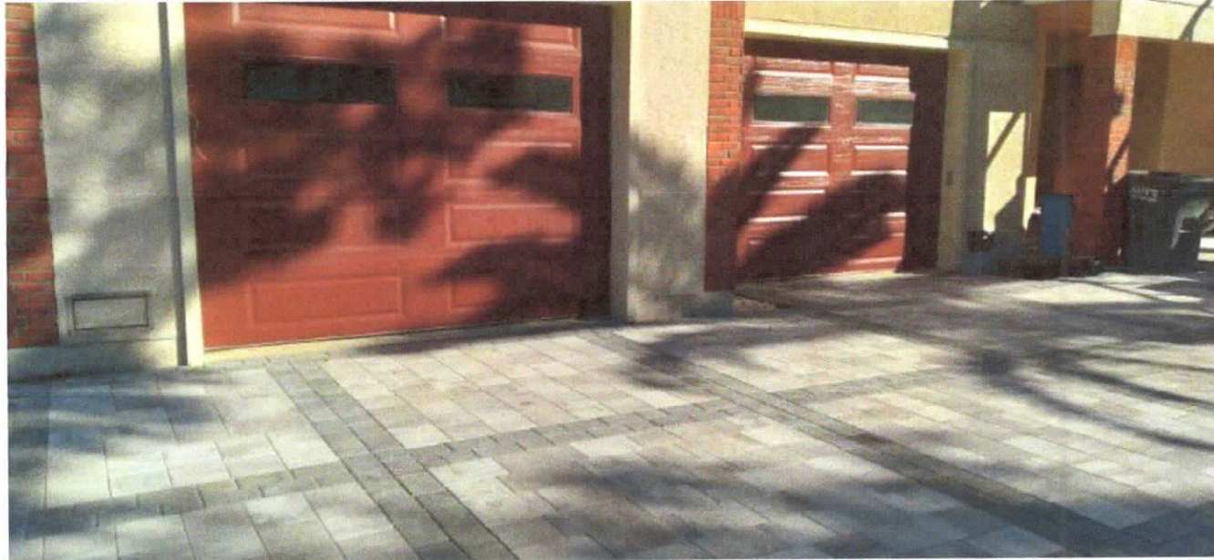
SMART VENT FLOOD VENT SOUTH SIDE 10-19-2022
