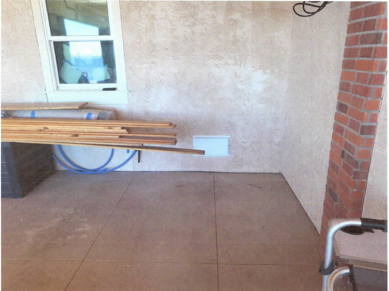
CRAWL SPACE DOOR SYSTEMS INC. FLOOD VENT 10-19-2022
