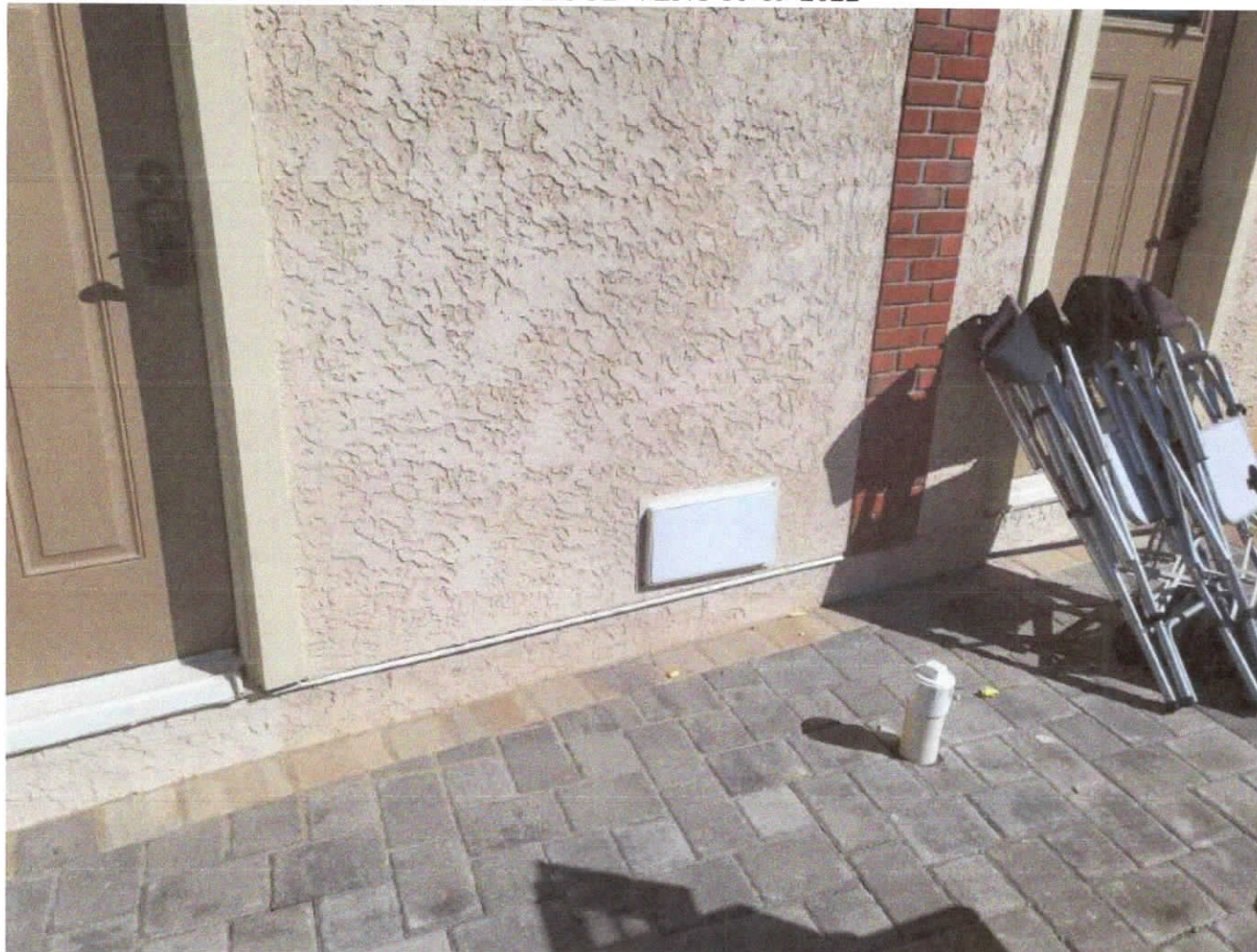
CRAWL SPACE DOOR SYSTEMS INC. FLOOD VENT 10-19-2022
