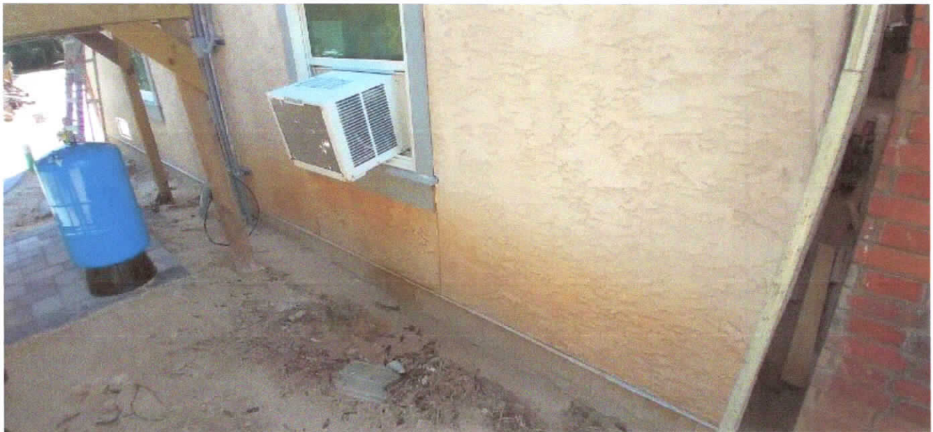
SMART VENT FLOOD VENT EAST SIDE 08-19-2022
